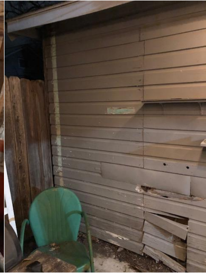
Rotting and patches throughout structure
