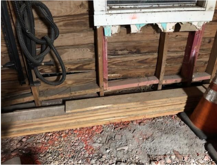
Neighboring tree (mature) is pushing through wall
